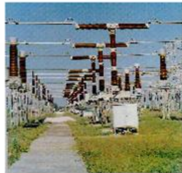
Live tank breaker (Courtesy BHEL)
