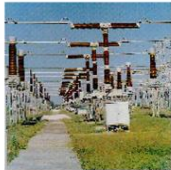
Live tank breaker (Courtesy BHEL)
